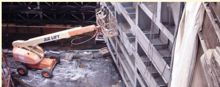
When repairs are finished, the Poe gates will be painted as were gates in this neighboring lock in 2009.
