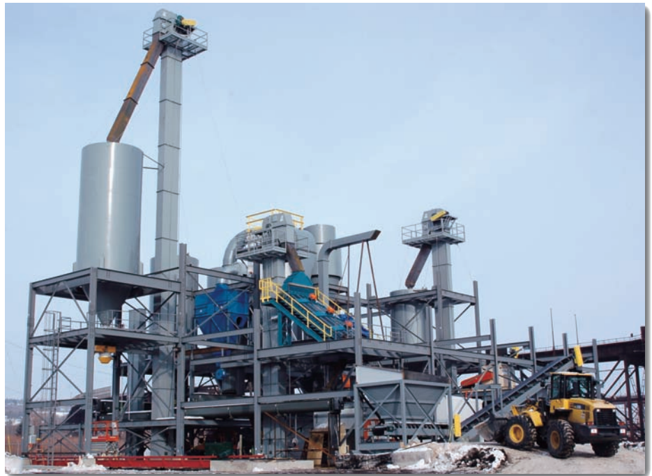
Who needs an exterior? Duluth Minerals got its processing equipment in place — and went to work uncovered. Operations now. 'Skin' later this year.
