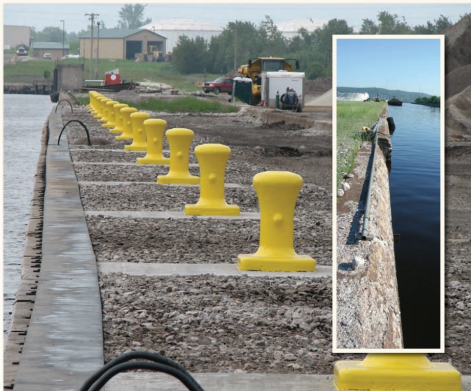
Once-crumbling dock walls at Hallett Dock No. 8 (inset) are being rehabilitated in a $3 million project.
