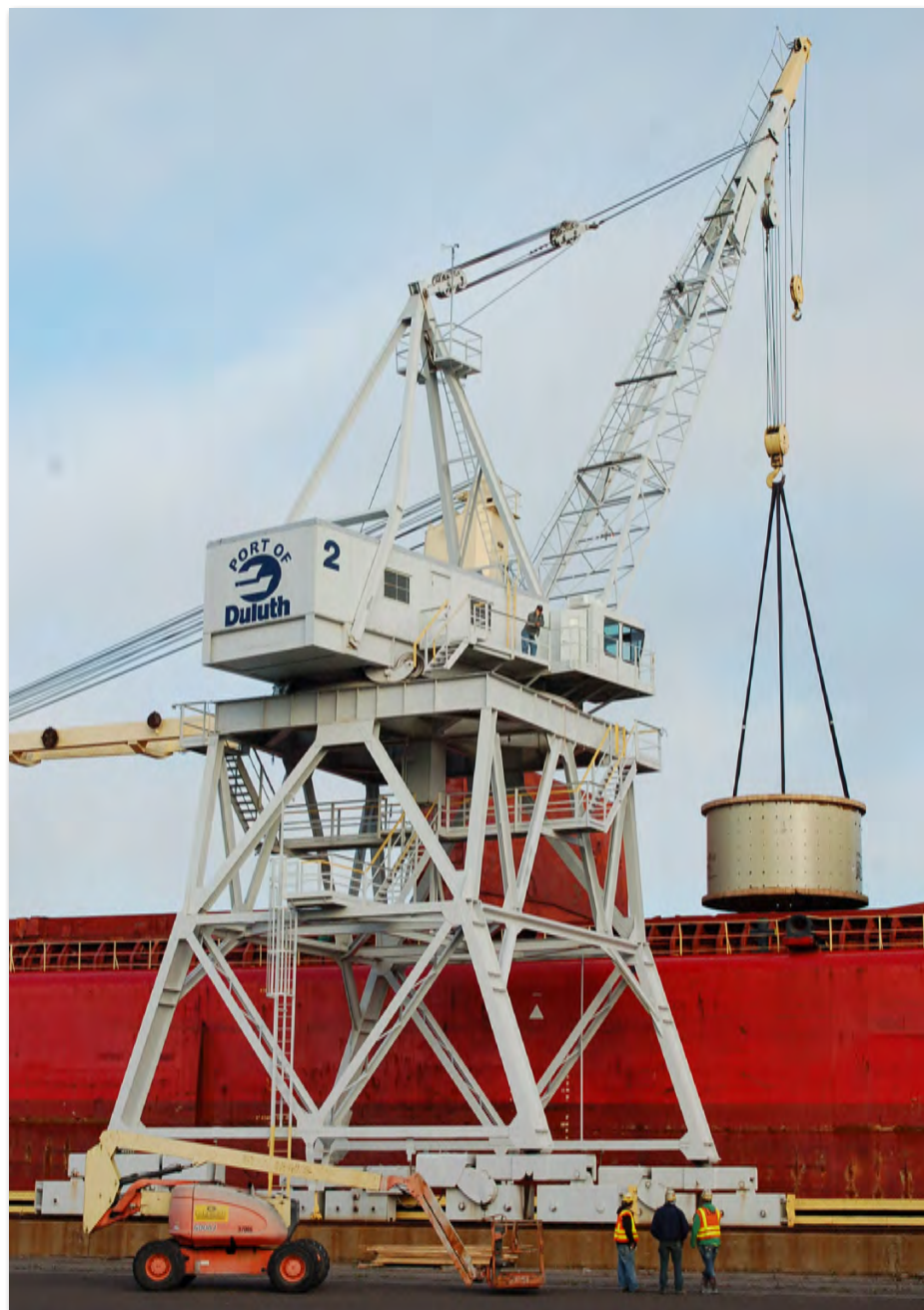
A ball mill shell is lifted from the Federal Maas at Duluth's Clure Public Marine Terminal. The shells are being installed in Magnetation's beneficiation plant near Grand Rapids, Minn.
