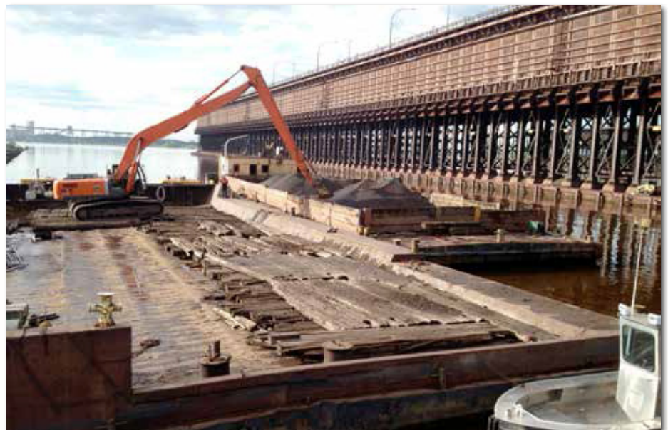
CN's Dock 6 will have a total of 3,600 feet of new coated sheet piling, on both sides of the dock.
