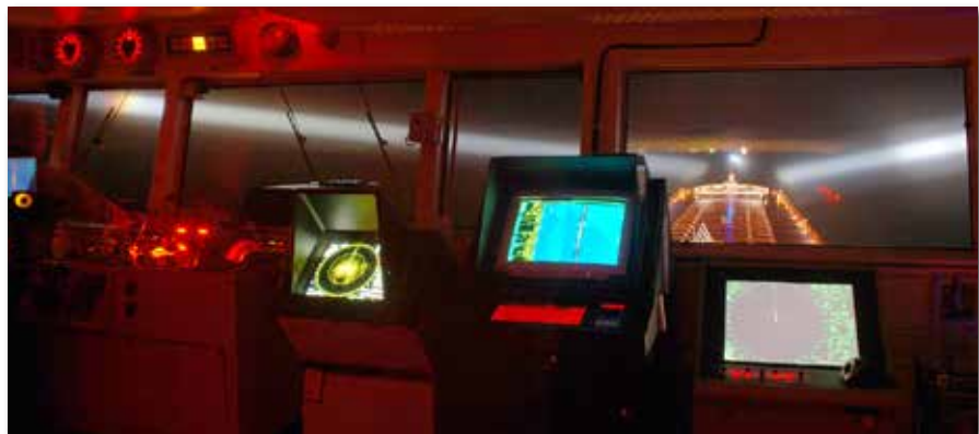
The pilothouse on a modern Great Lakes freighter is a marvel of navigation and weather technology.
