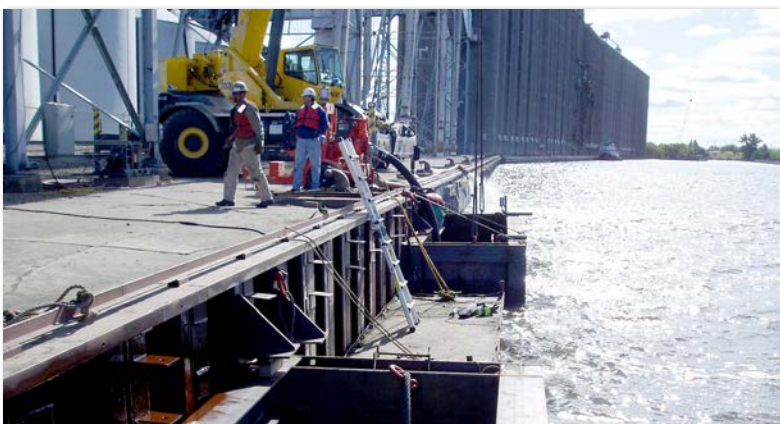
Marine Tech alternates two cofferdams to maintain high production on coating existing sheet pile at CHS where corrosion was not as severe as other locations. Cofferdams are leap-frogging down the dock to maximize time spent dewatering, sandblasting and coating.
