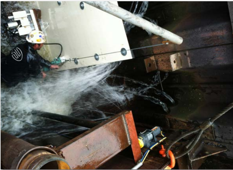
Dewatering and installing Aquapure coated steel plate on a dock rehab project. Notice the condition of existing sheet pile as water pours in through holes caused by corrosion.
