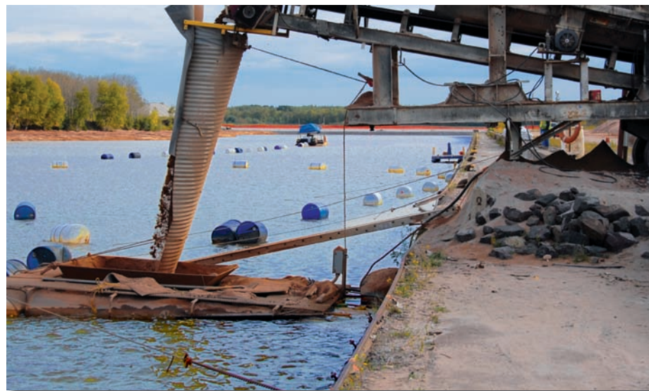
Hydraulic capping was key to the Stryker Bay mitigation process. Shown here is the sand feed conveyor connected to a hydraulic pump for sand capping delivery.
