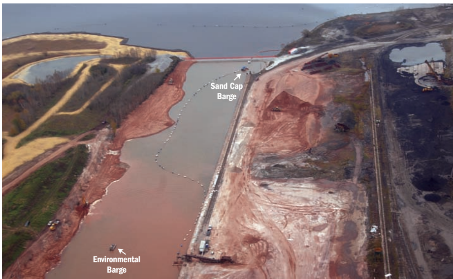
Slip 6 was turned into a Confined Aquatic Disposal area. Taken during capping operations, this photo shows Marine Tech’s environmental media barge in the foreground and its sand cap barge near the end of the slip.
