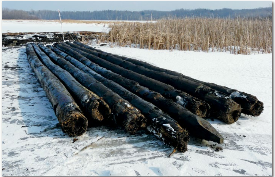
Here are just a few of the 460 pilings that were pulled from the bottom of the polluted Radio Tower Bay.
