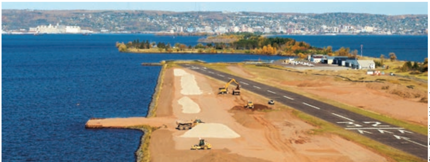
Heavy equipment smooths the way for runway relocation at Duluth’s Sky Harbor Airport. The project entered its final phase earlier this fall.
